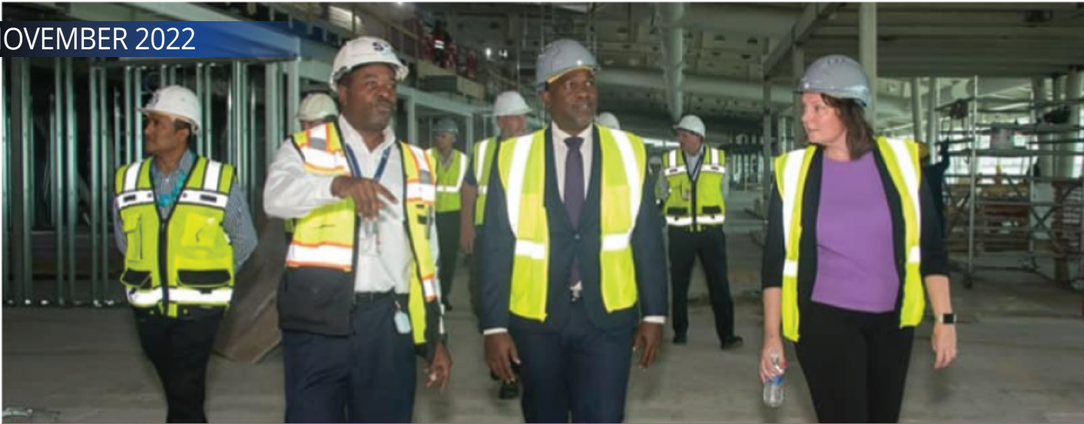
L to R Project Director of the Project Management Unit (PMU), Mirto Breell leads the tour at the former Departure Hall of the Airport Terminal Reconstruction Project as His Excellency Governor Ajamu Baly looks on.
